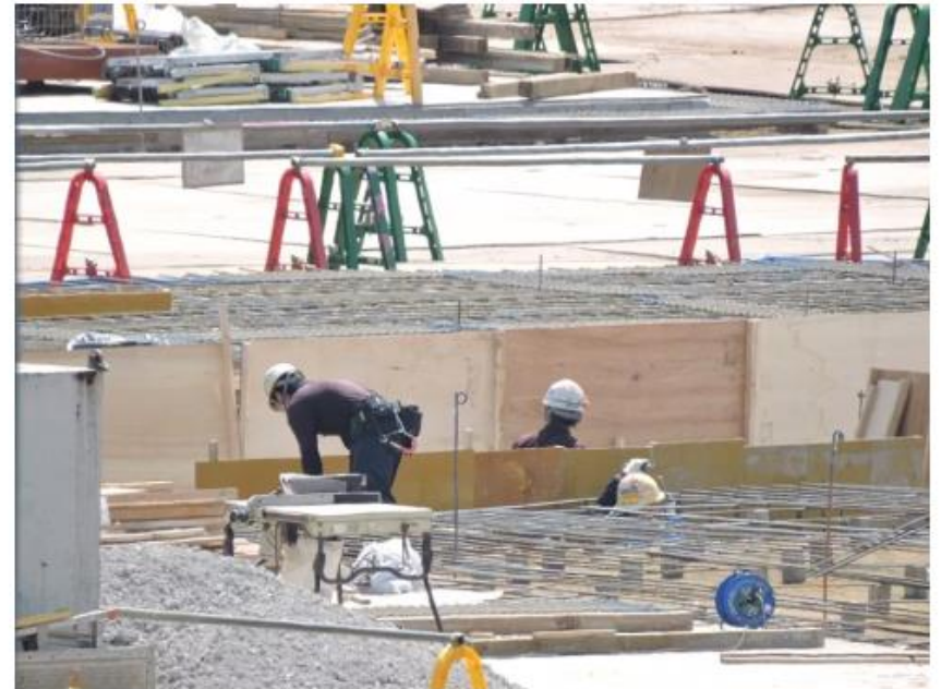
Construction site of the new Tokyo Olympic National Stadium. (Photo from the Japan Sports Council)
