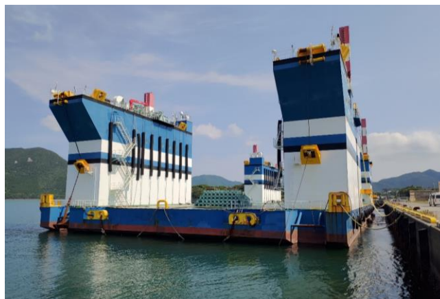
Photo 2. A special boat for offshore wind farm construction, 'Float Raiser' carries FOWT parts to the installation sites off the coast of Fukue Island, Goto City.
