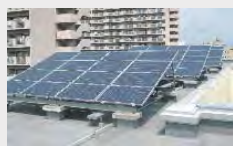
Photovoltaic power generation facility
