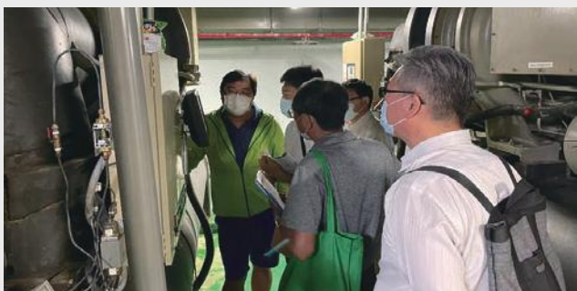
▲ Enterprise Zero Carbon Certification Counseling - Helping the shopping centers enhance their efficiency of energy-saving.
