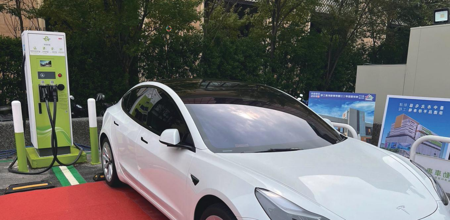
▲ The first fast charging station in the City's public parking lot has been opened in October 2023
