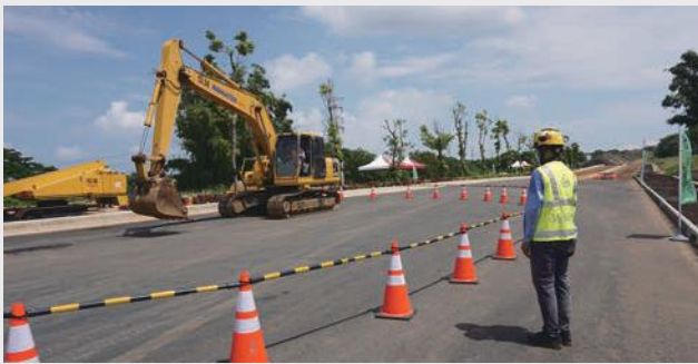
▲ Reduce the occurrence of worker collision accidents through the pre-sound function of the helmet sensor
