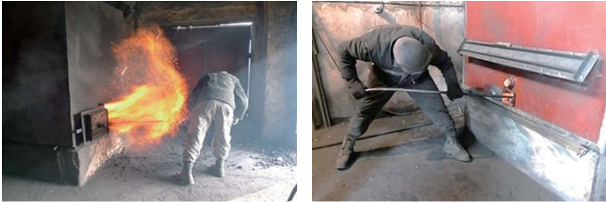
Figure 4.2 Controlling combustion by adjusting coal levels (left: before, right: after)
